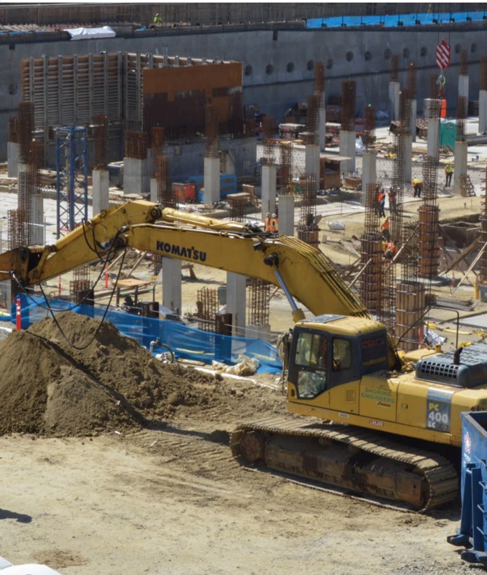
Construction workers lay the foundations for the new Long Beach City Hall and Port Administration Building in March 2017.
